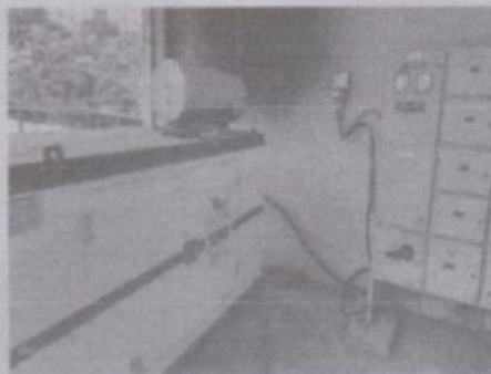
Fig(d): Diesel Generator
